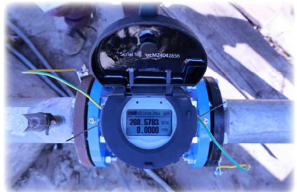
Recently Installed Digital Flow Meter at an Agricultural Well
